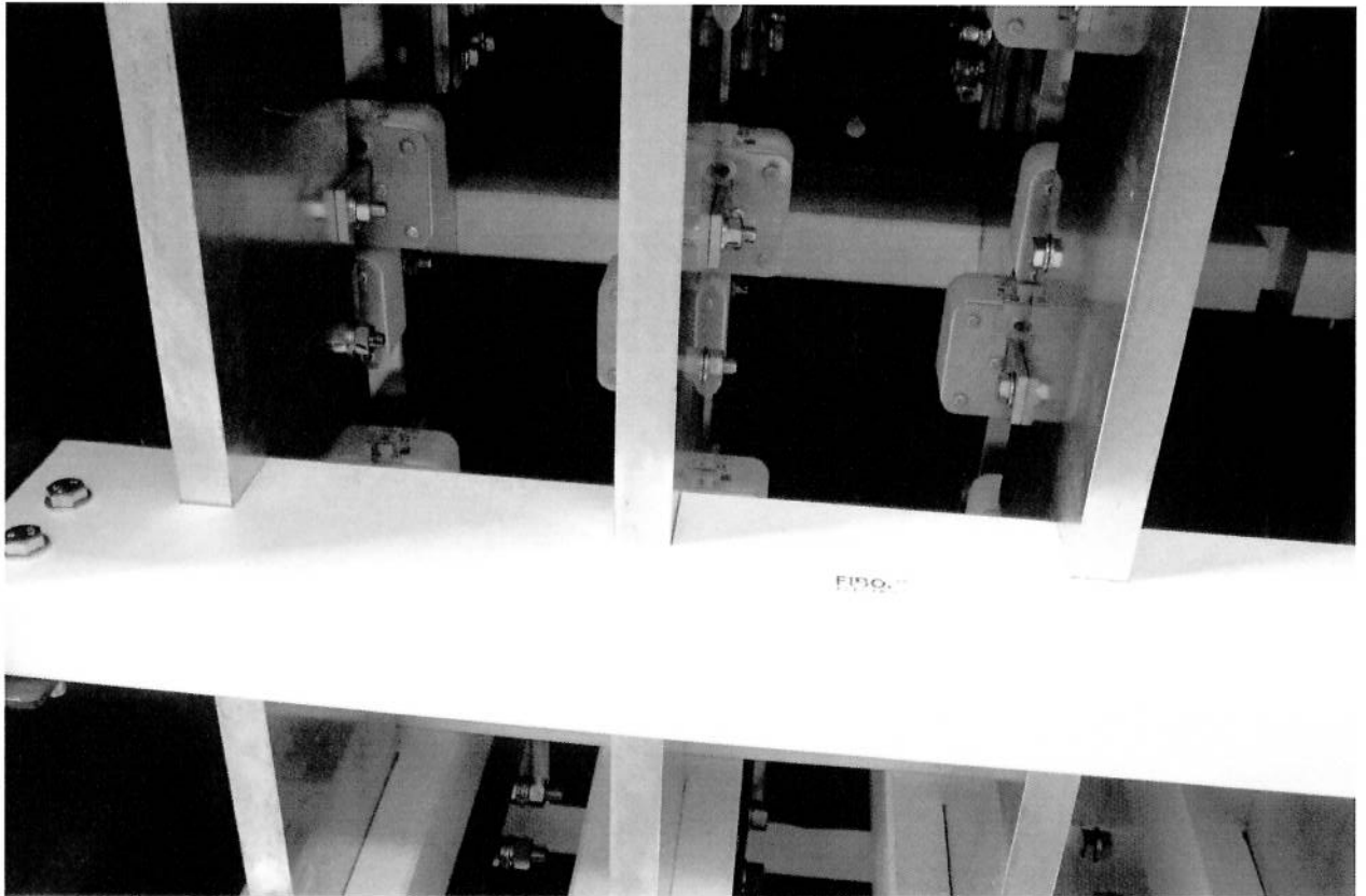
Photo 11037: Typical fuse-links fitted to assembly
